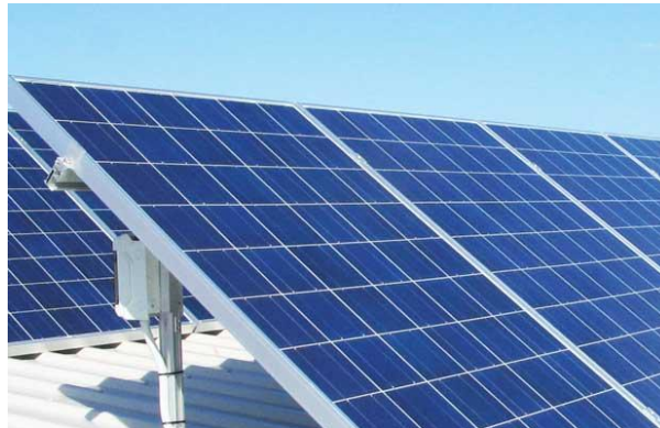
Figure 41. Photovoltaic solar panels
