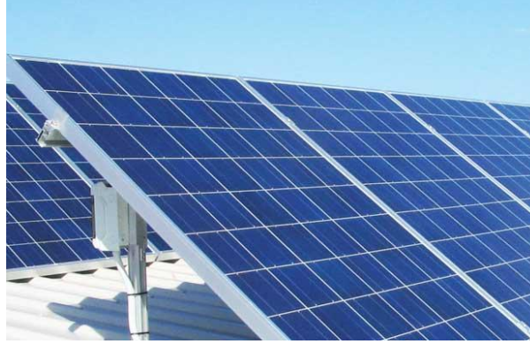
Figure 41. Photovoltaic solar panels
